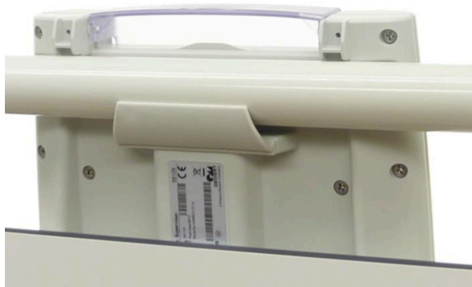
Figure 79. The nurse's control board installed at the end of the bed
